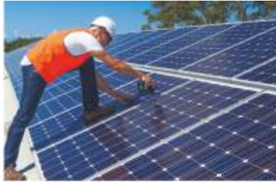
Requirements of the Solar industry
